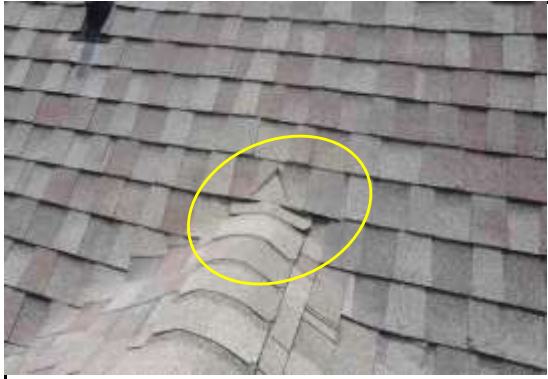
Flashing above ridge is missing fasteners.
