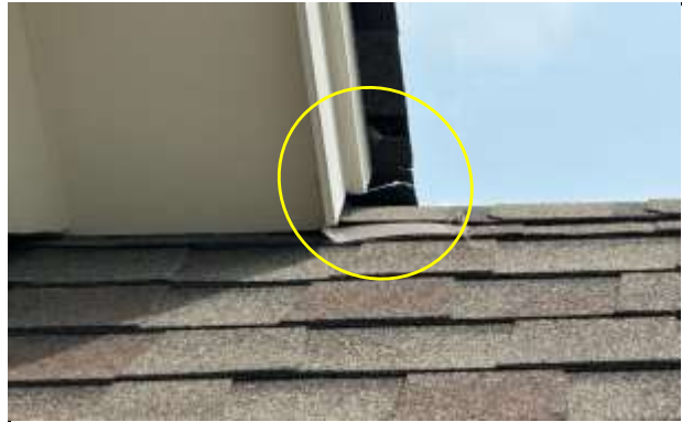
Shingle Condition - Shingle Damage/Missing Shingles/Granular Damage/Nail Pops/etc.
