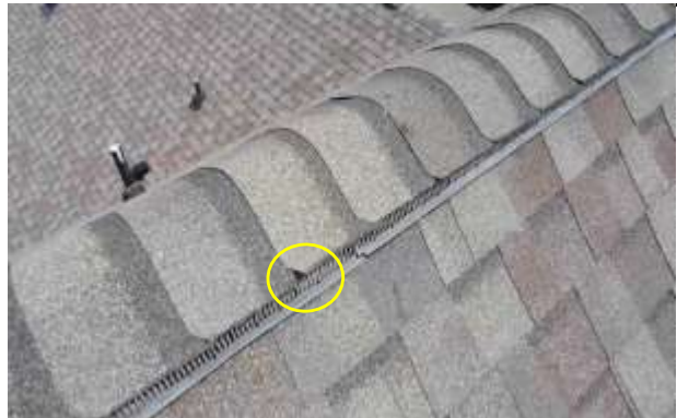
Shingle Condition - Shingle Damage/Missing Shingles/Granular Damage/Nail Pops/etc.
