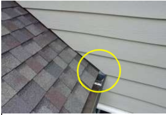
Flashing(s) Kickout - Kickout flashing(s) are missing where siding/shingles meet. Recommend professional contactor evaluate and install as necessary.
