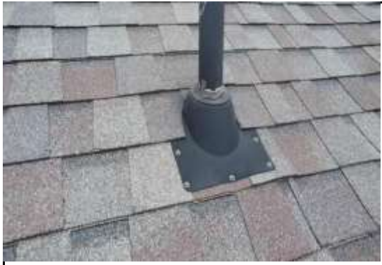
Plumbing Flashing - Plumbing flashings are in good shape. These flashings are recommended to be replaced every 8-10 years.
