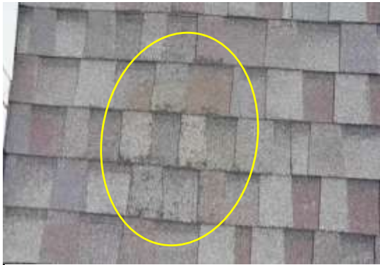
Shingle Condition - Shingle Damage/Missing Shingles/Granular Damage/Nail Pops/etc.
