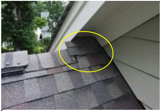
Flashing(s) at Shed Roof - Flashing are not properly installed at shed roof component.
