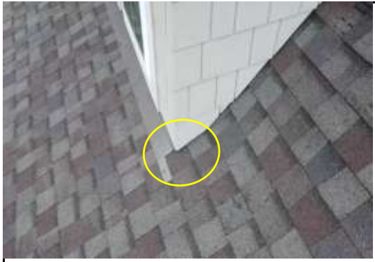
Flashing(s) Kickout - Kickout flashing(s) are missing where siding/shingles meet. Recommend professional contactor evaluate and install as necessary.
