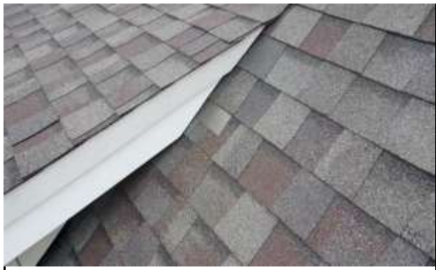
Flashing(s) at Shed Roof - Flashing are properly installed at shed roof component.
