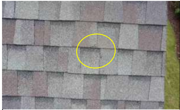
Shingle Condition - Shingle Damage/Missing Shingles/Granular Damage/Nail Pops/etc.
