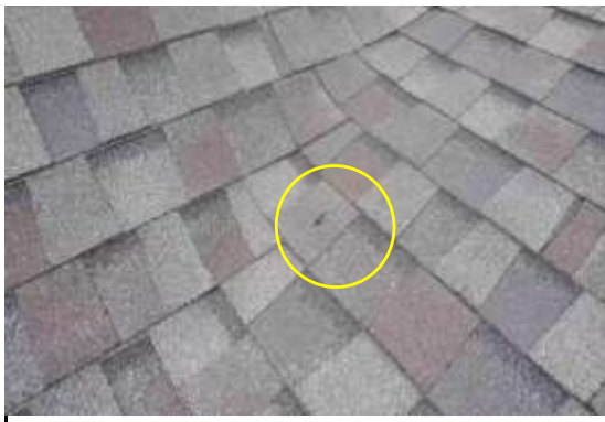
Shingle Condition - Observed nails/construction debris on the roof. Loose debris/nails can cause personal injury.
