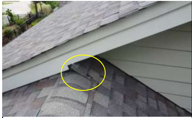
Flashing(s) at Shed Roof - Flashing are not properly installed at shed roof component.
