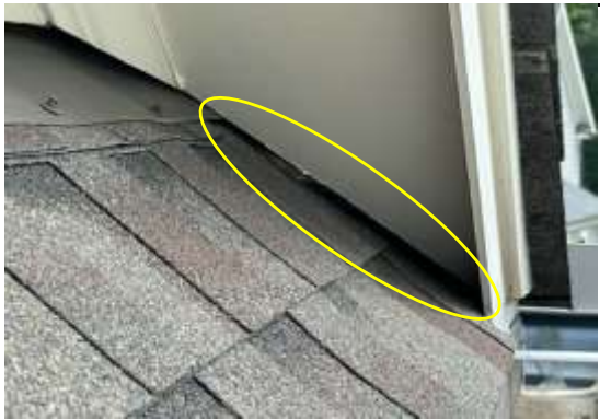
The gap between the soffit and roof shingles creates an opening into the attic for pests. Typically, flashing is installed in this area to seal off the attic.
