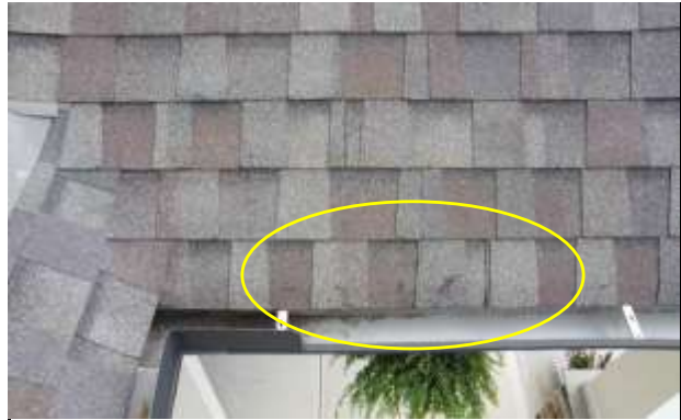
Shingle Condition - Shingle Damage/Missing Shingles/Granular Damage/Nail Pops/etc.
