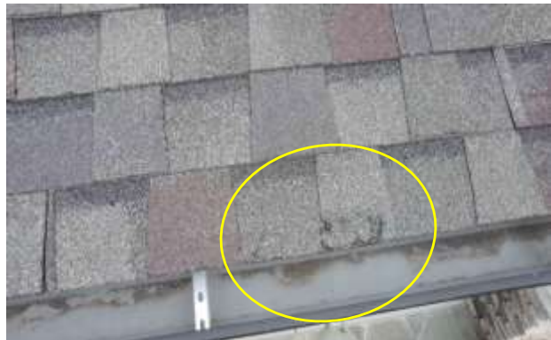
Shingle Condition - Shingle Damage/Missing Shingles/Granular Damage/Nail Pops/etc.
