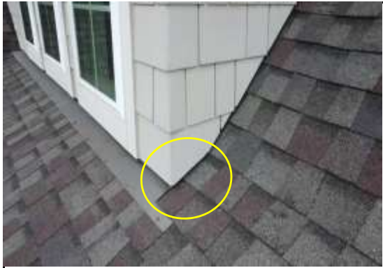
Flashing(s) Kickout - Kickout flashing(s) are missing where siding/shingles meet. Recommend professional contactor evaluate and install as necessary.
