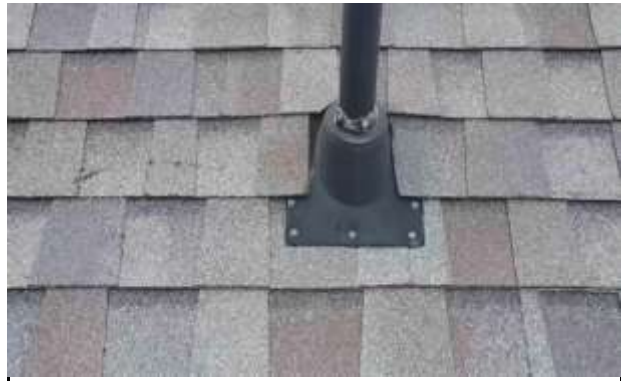
Plumbing Flashing - Plumbing flashings are in good shape. These flashing are recommended to be replaced every 8-10 years.
