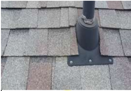
Plumbing Flashing - Plumbing flashings are in good shape. These flashing are recommended to be replaced every 8-10 years.
