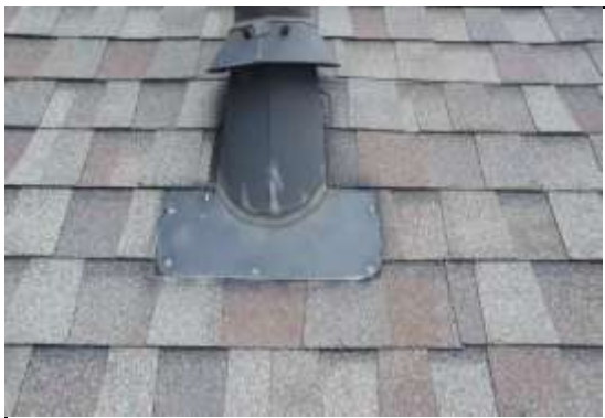
Mechanical Flashings - Mechanical flashings are in good shape. These flashings are recommended to be replaced every 8-10 years.
