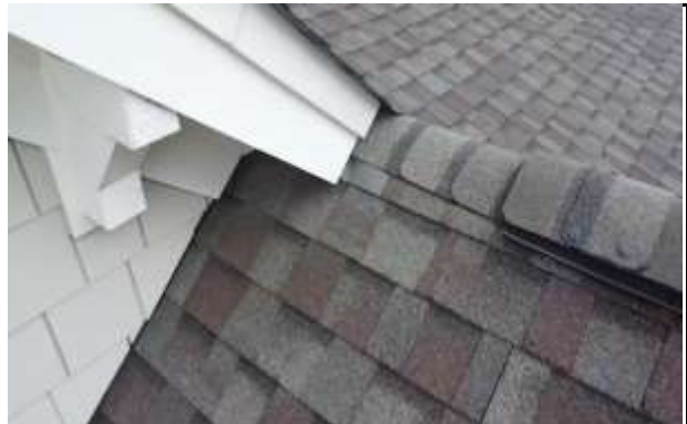
Flashing(s) at Overhang Returns - Flashings are properly installed and attachment is sealed properly
