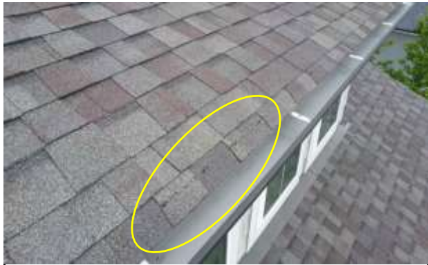
Shingle Condition - Shingle Damage/Missing Shingles/Granular Damage/Nail Pops/etc.
