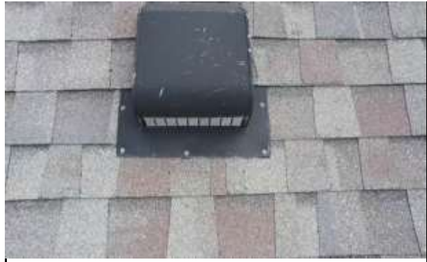
Mechanical Flashings - Mechanical flashings are in good shape. These flashings are recommended to be replaced every 8-10 years.
