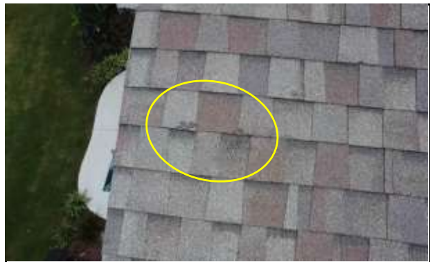
Shingle Condition - Shingle Damage/Missing Shingles/Granular Damage/Nail Pops/etc.
