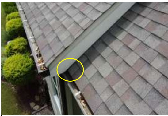
Flashing(s) Kickout - Kickout flashing(s) are missing where siding/shingles meet. Recommend professional contactor evaluate and install as necessary.
