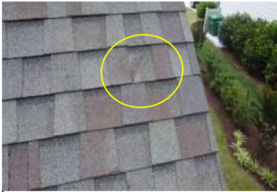
Shingle Condition - Shingle Damage/Missing Shingles/Granular Damage/Nail Pops/etc.
