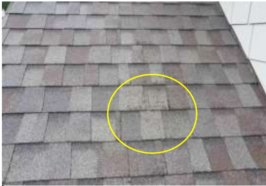
Shingle Condition - Shingle Damage/Missing Shingles/Granular Damage/Nail Pops/etc.
