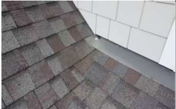
Flashing(s) at Overhang Returns - Flashings are properly installed and attachment is sealed properly
