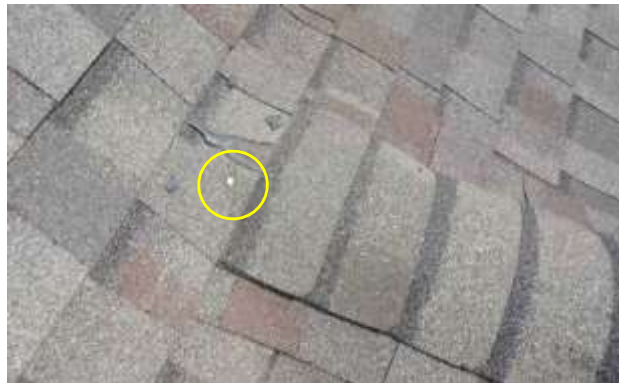
Shingle Condition - Sealant missing/deteriorated from nail heads.
