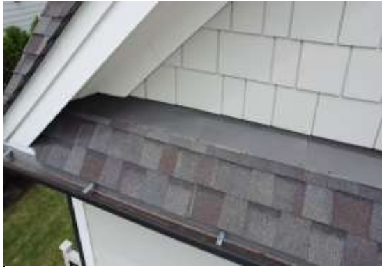
Flashing(s) at Overhang Returns - Flashings are properly installed and attachment is sealed properly
