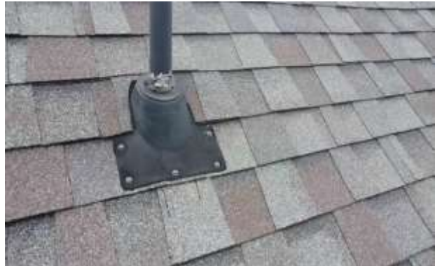
Plumbing Flashing - Plumbing flashings are in good shape. These flashing are recommended to be replaced every 8-10 years.
