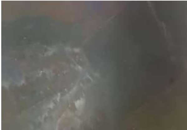
Flue - Flue joints are in typical conditions Photo 19 LOG
