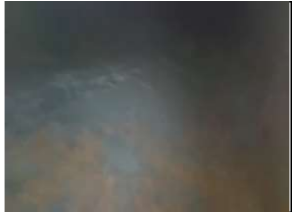
Flue - Flue joints are in typical conditions Photo 26 LOG
