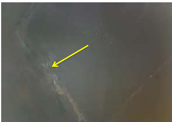
Flue - Soot Deposits - There is an accumulation of soot/debris in the flue. Soot deposits increase the risk of flue fire. Recommend regular cleaning. Photo 15 INFO
