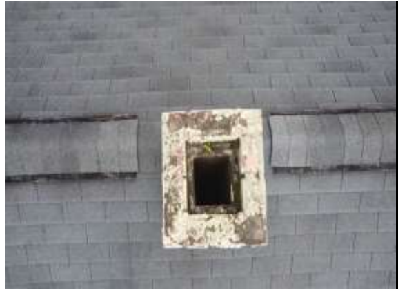
Old flue/chimney - There is a second chimney on the home that used to serve an old gas/oil fired furnace system or water heater. These flues commonly have openings into the crawlspace. The open cap can allow water/pests/debris into the Photo 32 LOG
