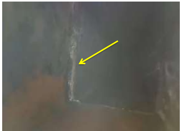
Flue - Soot Deposits - There is an accumulation of soot/debris in the flue. Soot deposits increase the risk of flue fire. Recommend regular cleaning. Photo 24 LOG
