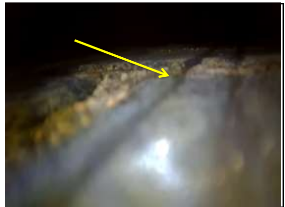
Smoke Chamber - Signs of moisture running through the area.
