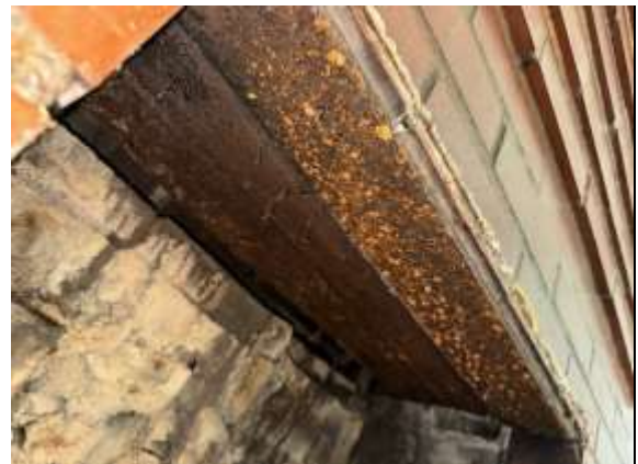
The fireplace lintel is rusted and shows some signs of deterioration. Service/repair is needed to prevent further deterioration.
