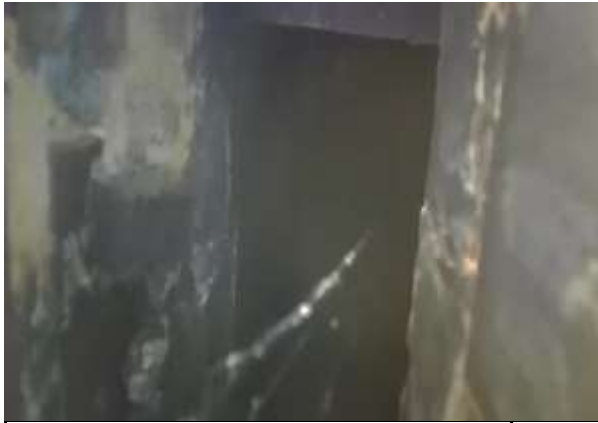
Flue - Flue joints are in typical conditions Photo 13 LOG
