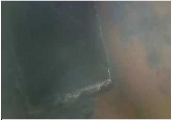
Flue - Flue joints are in typical conditions Photo 25 LOG
