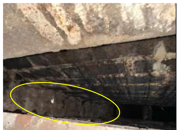
Smoke Chamber - Mortar deterioration is present in the smoke chamber. This can allow heat to pass through the wall and can result in loose bricks.
