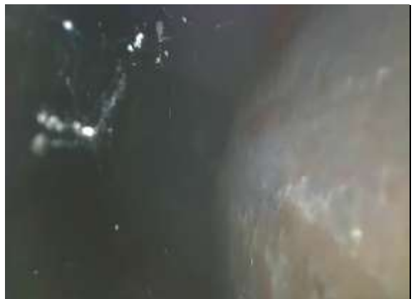
Flue - Flue joints are in typical conditions Photo 22 LOG
