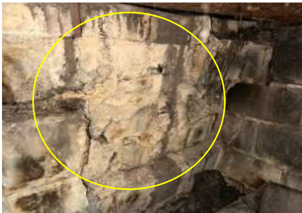
Firebox - Firebrick mortar deterioration present. This can allow heat to pass through the firebox wall and can result in loose bricks. Photo 5 LOG
