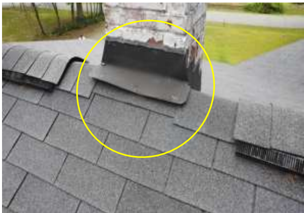
Chimney Penetration Flashing - Deteriorated/Lifting up. This can result in moisture penetration and damage. Photo 35 LOG
