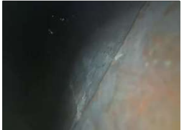
Flue - Flue joints are in typical conditions Photo 20 LOG
