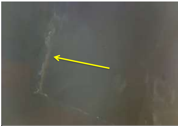
Flue - Soot Deposits - There is an accumulation of soot/debris in the flue. Soot deposits increase the risk of flue fire. Recommend regular cleaning. Photo 17 INFO
