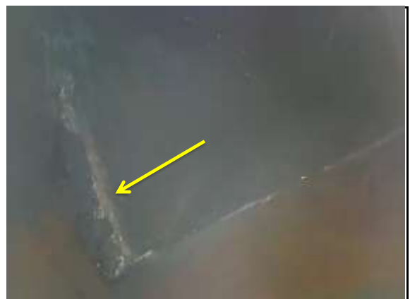
Flue - Soot Deposits - There is an accumulation of soot/debris in the flue. Soot deposits increase the risk of flue fire. Recommend regular cleaning. Photo 16 INFO
