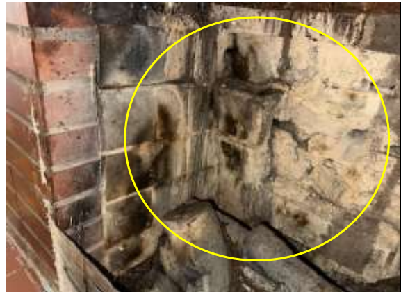
Firebox - Firebrick mortar deterioration present. This can allow heat to pass through the firebox wall and can result in loose bricks. Photo 4 INFO
