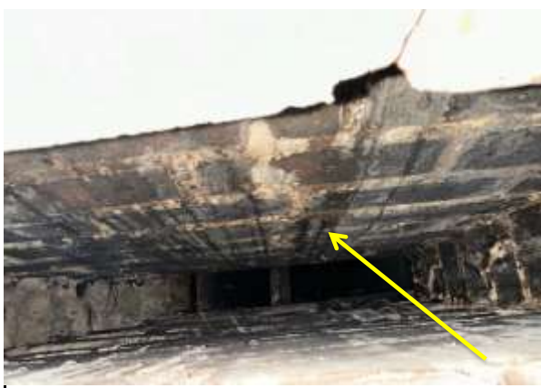
Smoke Chamber - Signs of moisture running through the area.
