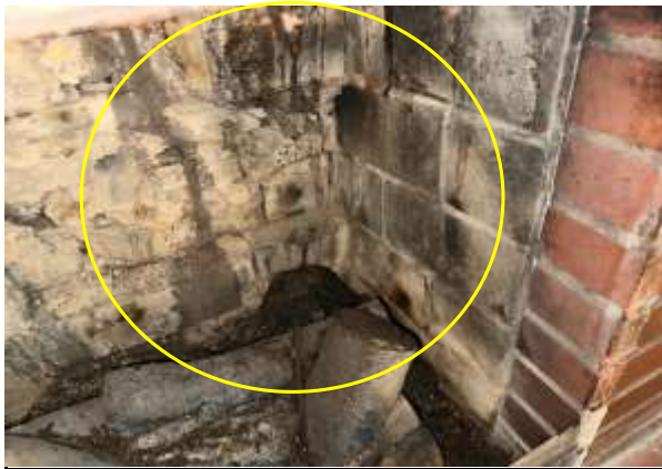
Firebox - Firebrick mortar deterioration present. This can allow heat to pass through the firebox wall and can result in loose bricks.
