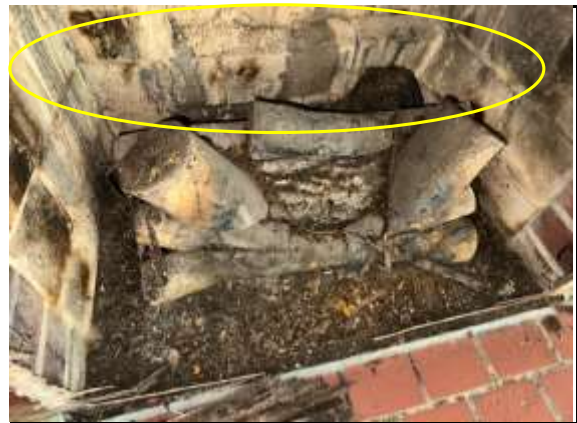
Firebox - Firebrick mortar deterioration present. This can allow heat to pass through the firebox wall and can result in loose bricks. Photo 6 LOG
