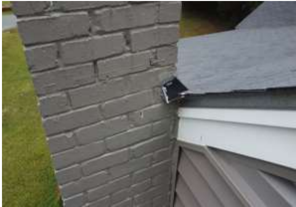
Chimney Penetration Flashing - Normal condition, typical installation in this area. Photo 31 LOG
