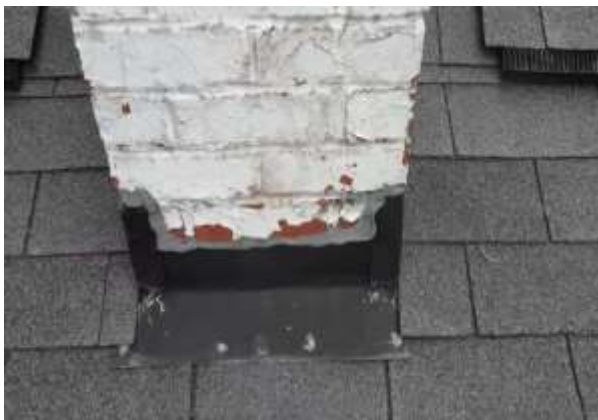
Chimney Penetration Flashing - Normal condition, typical installation in this area. Photo 33 LOG
