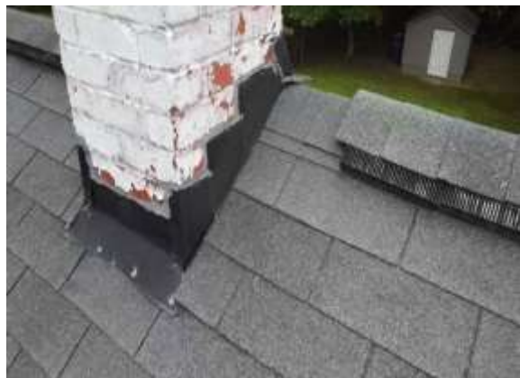
Chimney Penetration Flashing - Normal condition, typical installation in this area. Photo 34 LOG
