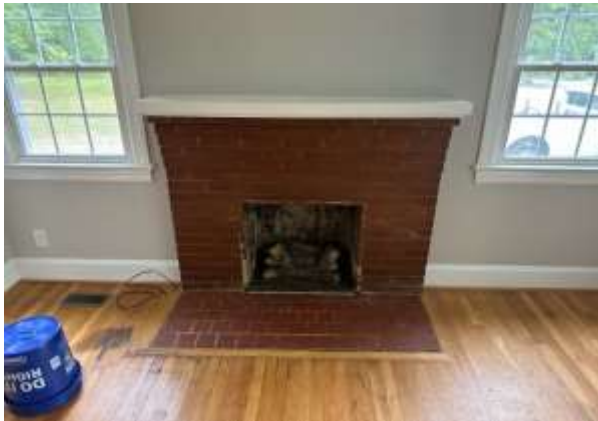
Fireplace/firebox Photo 3 INFO
