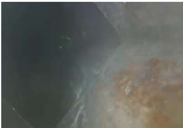
Flue - Flue joints are in typical conditions Photo 21 LOG
