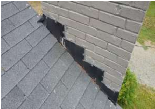
Chimney Penetration Flashing - Normal condition, typical installation in this area. Photo 29 LOG
