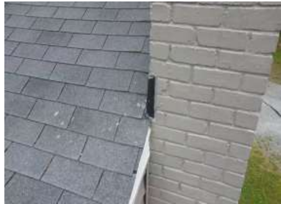
Chimney Penetration Flashing - Normal condition, typical installation in this area. Photo 30 LOG
