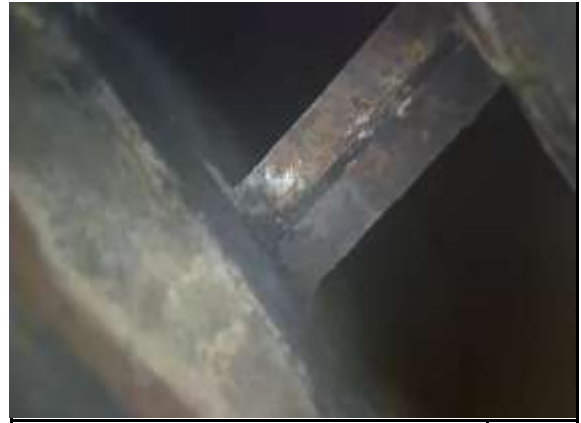
Flue - Flue joints are in typical conditions Photo 14 LOG
